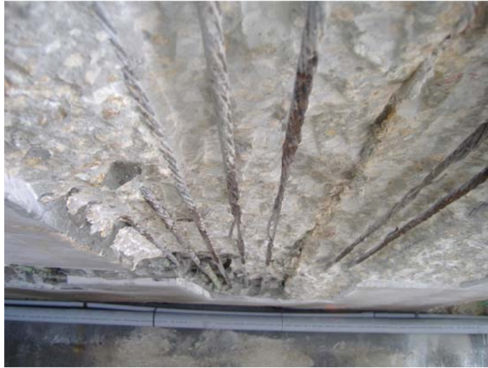
Figure 2.6 - Areas with spalled concrete and damaged strands
