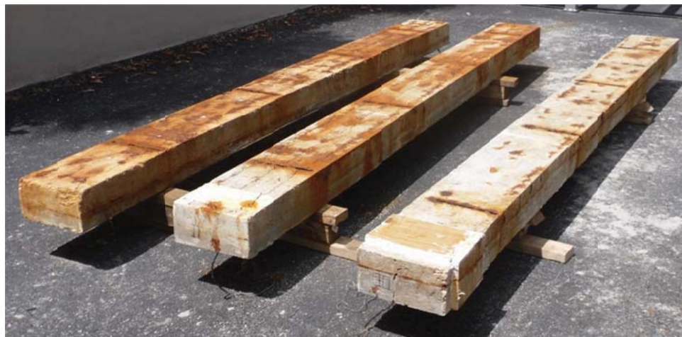
Figure 4.8 - Visual inspection after corrosion (B1 to B3)
