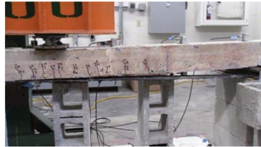
(b) Delamination B2
